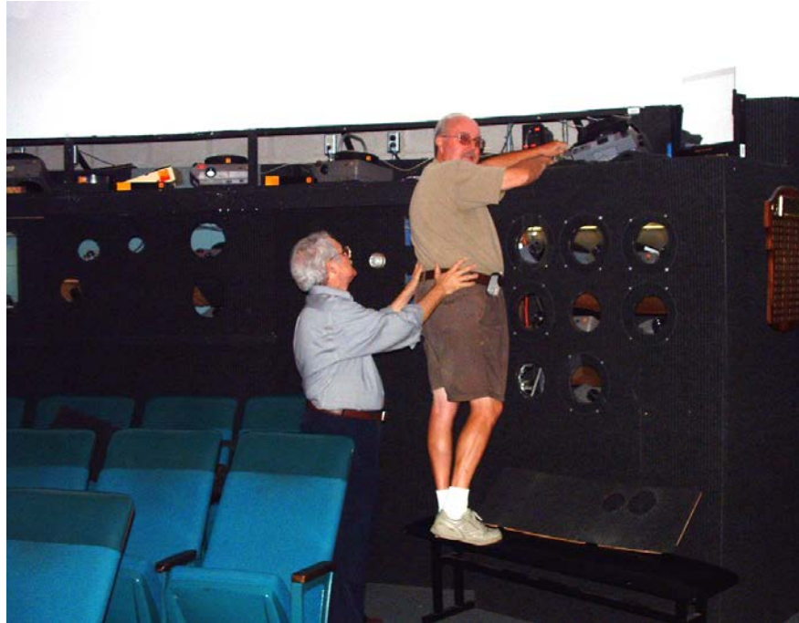
Figure 32 - Installing the final cabling in the ceiling of the MOAS Planetarium from the SRT Controller to the Computer Control Station
