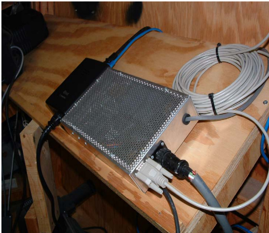
Figure 43 - The "iboot" Remote Power Controller supporting the SRT Antenna Driver System and Receiver.
