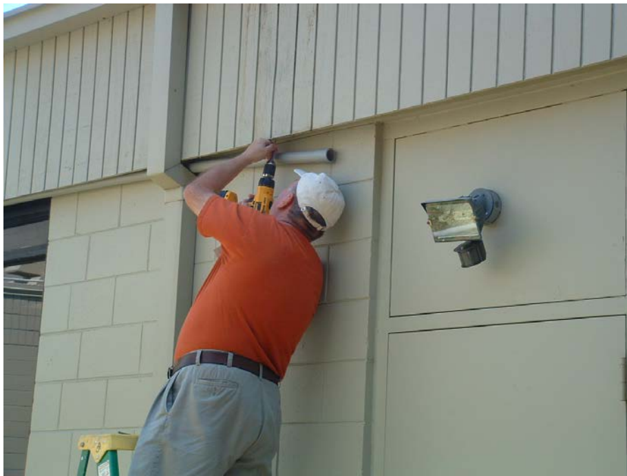
Figure 28 - Installing Conduit to carry the SRT Control and Data Cables under the Overhang at the Daytona Museum of Arts and Science
