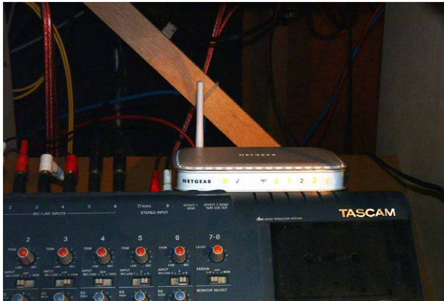
Figure 42 - The network router installed in the SRT equipment rack
