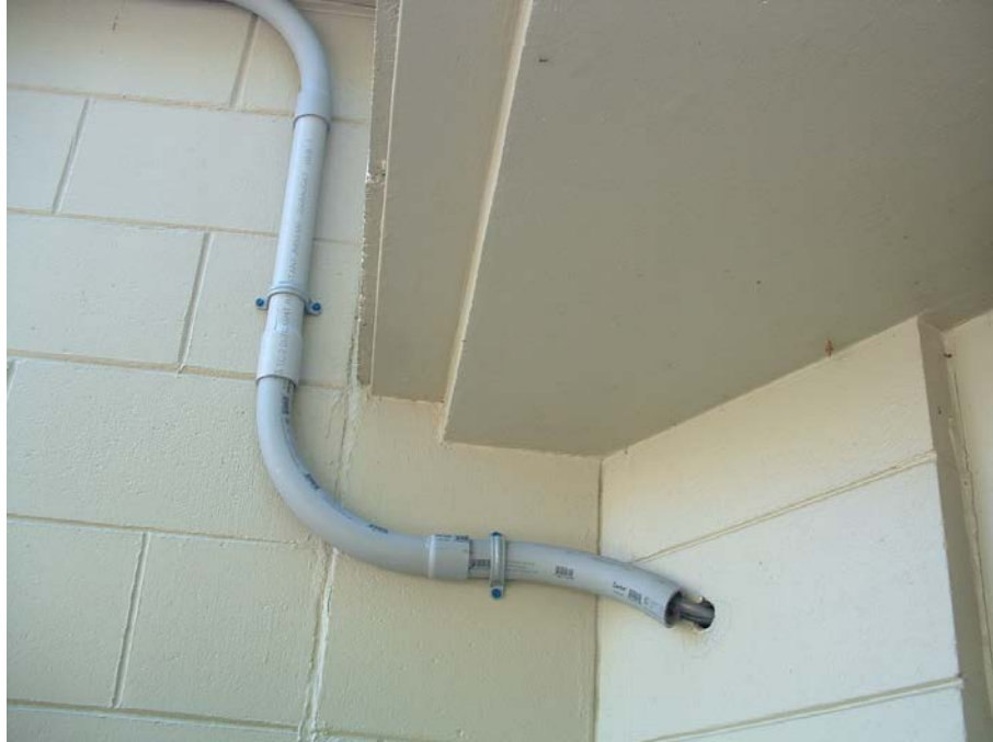
Figure 30 - The Control Cable Conduits where they enter the wall of the Planetarium
