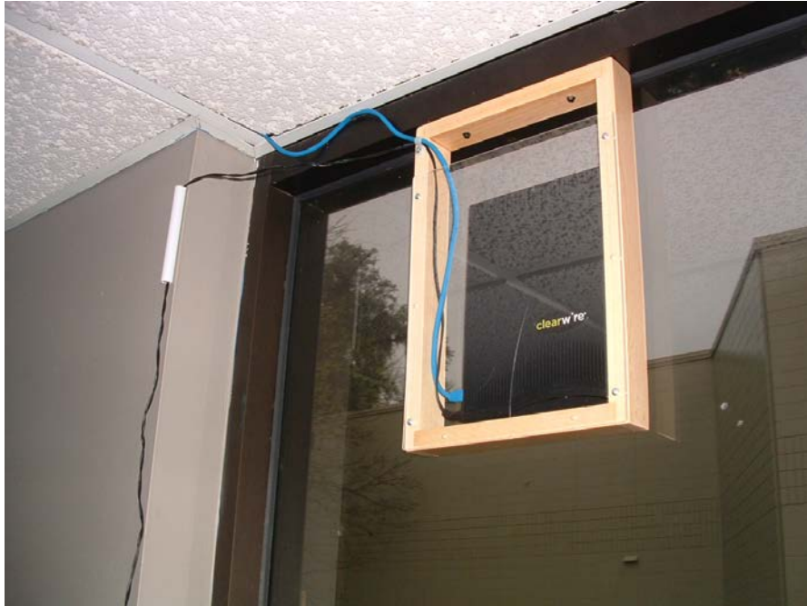
Figure 41 - The Clearwire Ethernet Modem installed in a window of the Planetarium Wing of the museum
