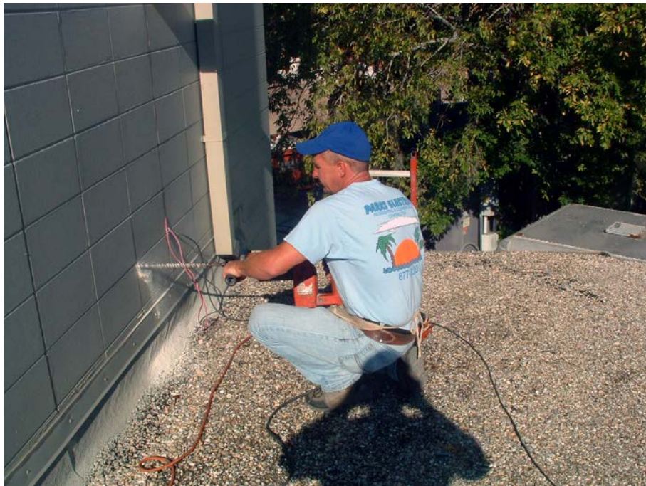
Figure 45 - The Electrical Contractor boring the hole for the floodlight wiring through the exterior wall of the Planetarium
