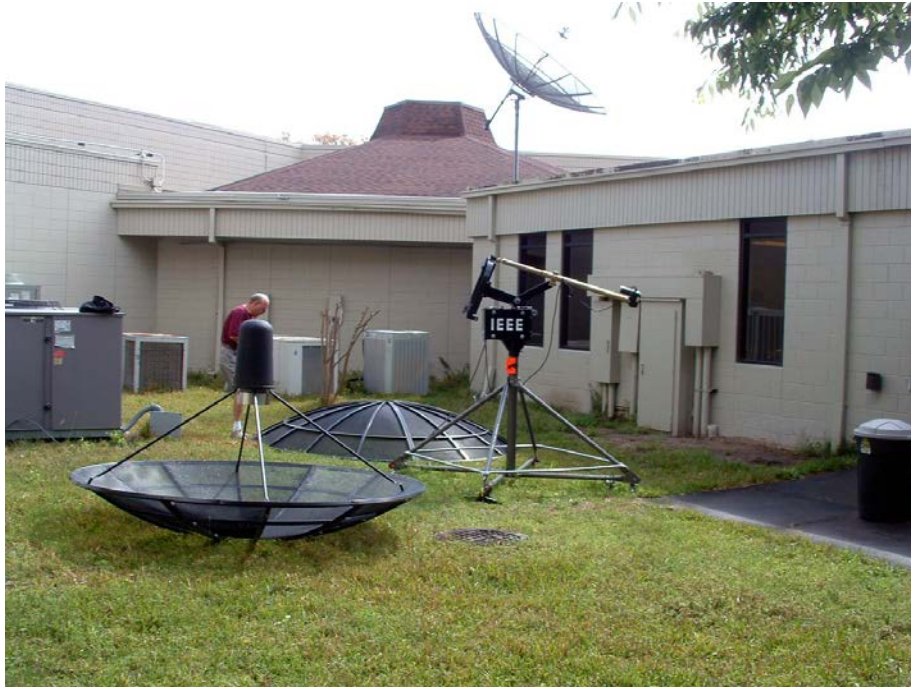
Figure 19 - The Removal of the 7.5 Foot Parabolic Reflector and the Assembly of the 10 Foot Parabolic Reflector
