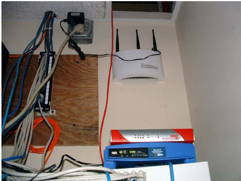
Figure 37 - The Hawkings 300N Router installed in the wiring closet in the damaged wing of the museum
