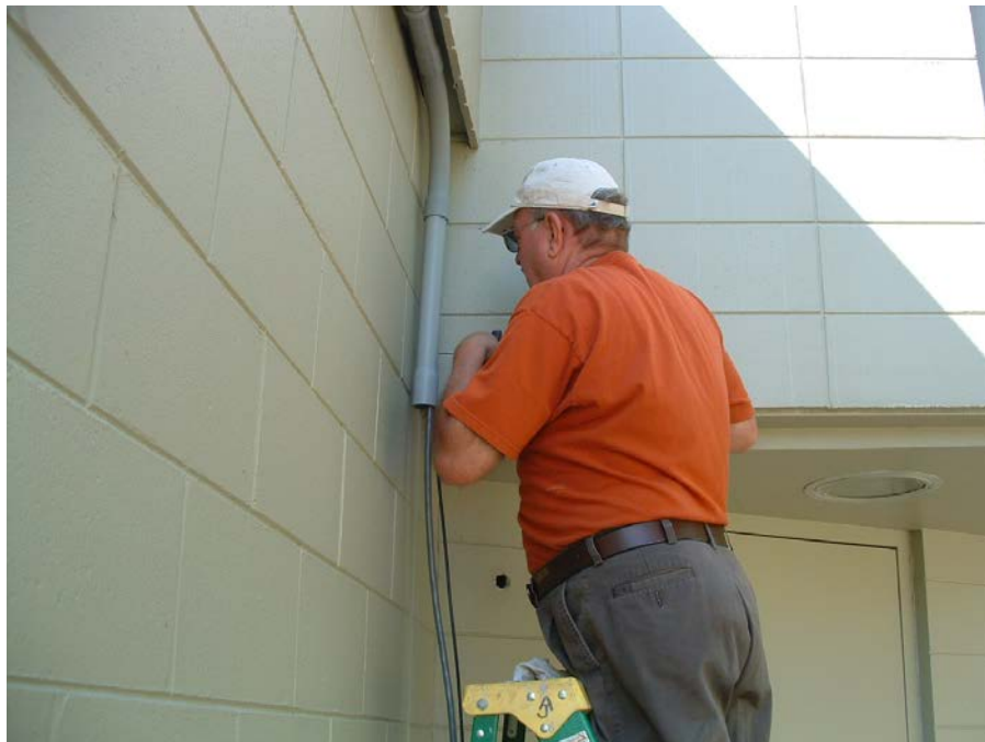
Figure 29 - Al Jusko working on the final segment of the Outside Conduit and SRT Control and Data Cables
