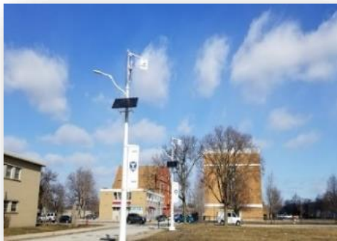
ARIS Lights: Partnered with CHA, CPD, CPS, and ARIS Wind to install solar/wind/battery powered lighting units
